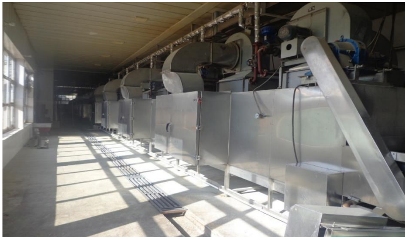
Fig. 2. General view of a convective dryer.
